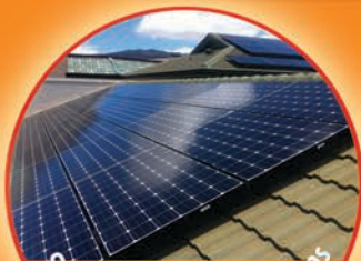
Solar Roof Top Solutions
