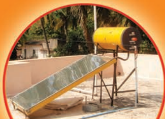
Solar Water Heaters
